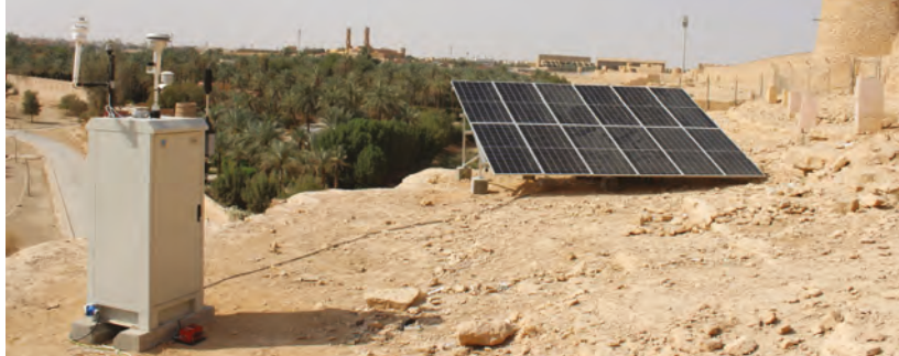
Saudi Arabia Installed Fenceline monitoring station with renewable energy power source
